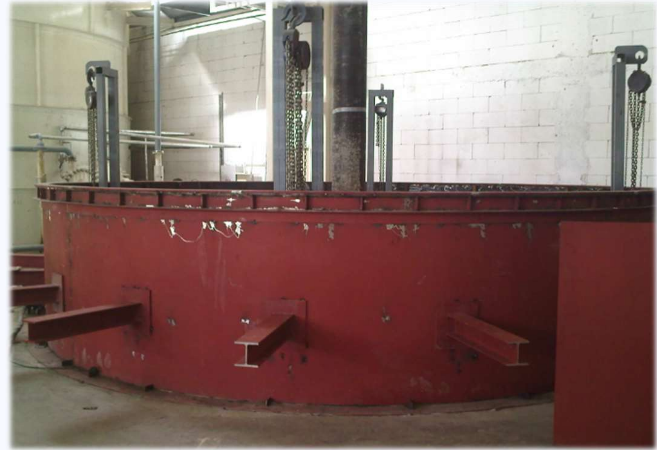
Sludge Tank- Bilecik Ytong (Xella Project)
